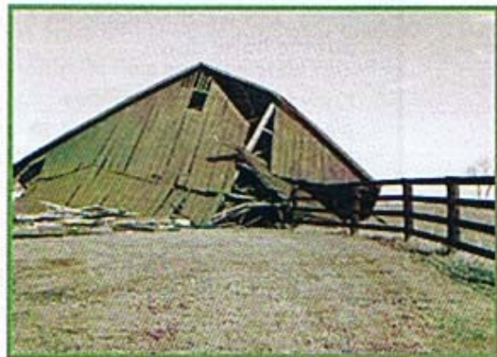
Centaur fence in Kentucky that withstood damaging winds as well as the weight of a barn.
